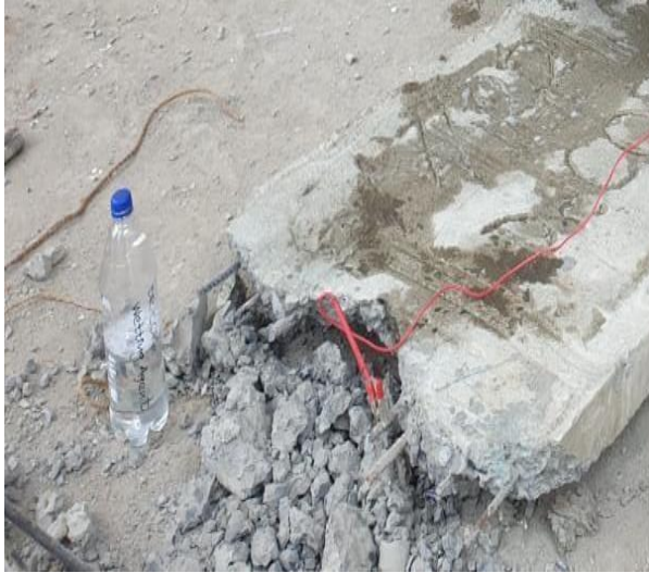
Figure 11: Specimen broken from side to exposed rebars
