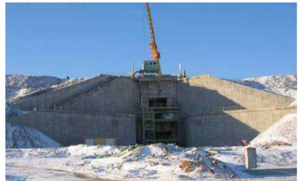
Crusher Plant (Crusher walls)
