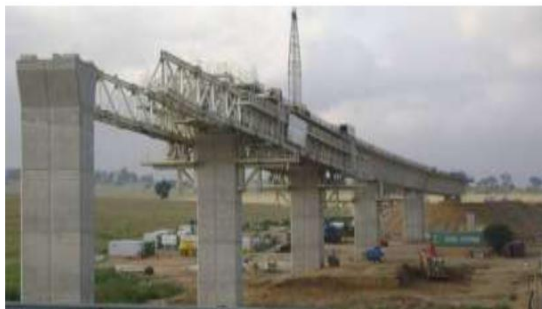
Figure 1 : File photo of viaduct showing launching girders resting on brackets attached to piers
