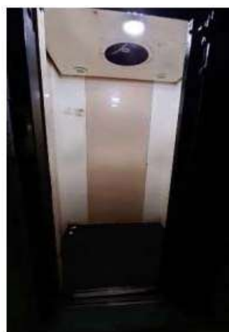
Fig 1 - Lift car which is insufficient for wheelchair accessibility(0.9x0.9m)
